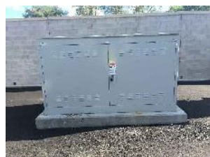
INDICATIVE PRIMARY METERING CABINET
